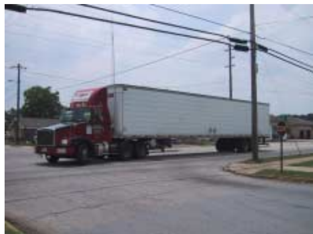
Faded Stop Line and Center Line Marking at Furnace Street and West Avenue
